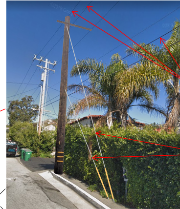
NEW 50 FT RISER POLE W/ GUY ANCHORS
