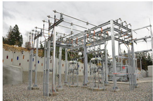
Electrical substations are vital facilities to ensure that electrical service is safe and reliable. Image from Paul Chernikhowsky.
