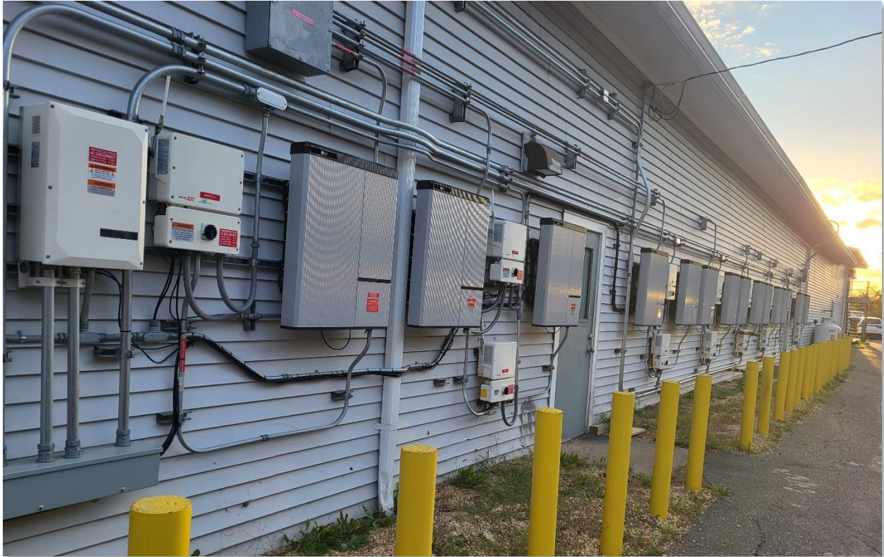
FIGURE 18: EXAMPLE MUNICIPAL WALL-MOUNTED BESS (APPROXIMATELY 280 KWH)
