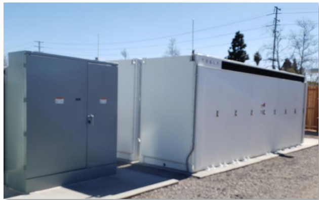
FIGURE 17: EXAMPLE GROUND MOUNT BESS (APPROXIMATELY 1500 KWH)
