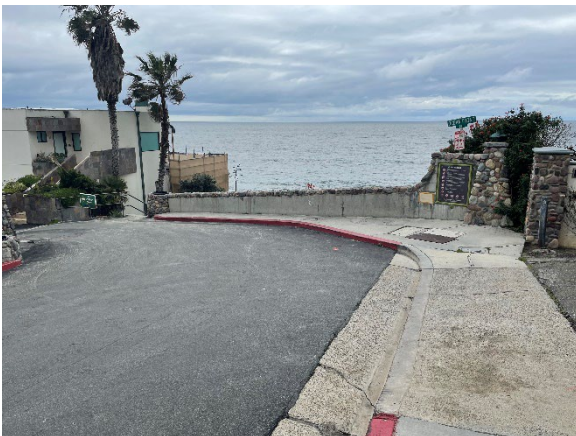
Photograph 3: View of concrete wall at top of Cleo Street beach access stairs, looking west (Stantec, March 2023)
