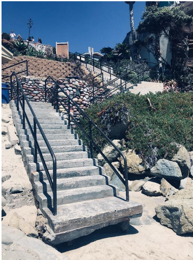
Photo 2: View of existing Cleo Street beach access looking from beach to top of stairs.
